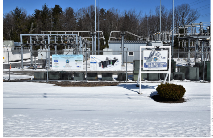
Massachusetts is one of several states that have implemented policies to spur energy storage development. Above, the state’s first utility-scale energy storage facility in Sterling, which stores electricity from a nearby solar array.
