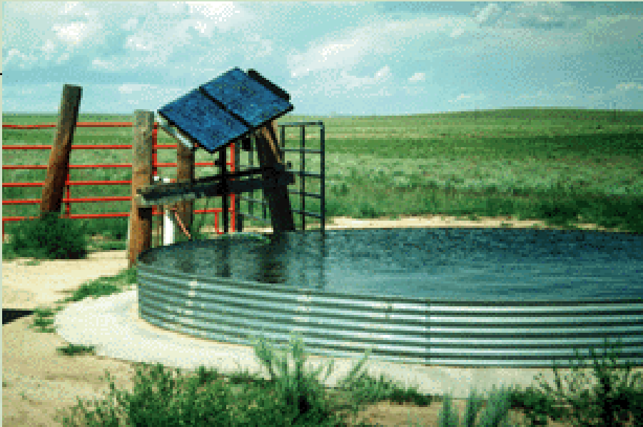
Solar power pumps water on this Colorado ranch. Photo: K.C. Electric, NREL
