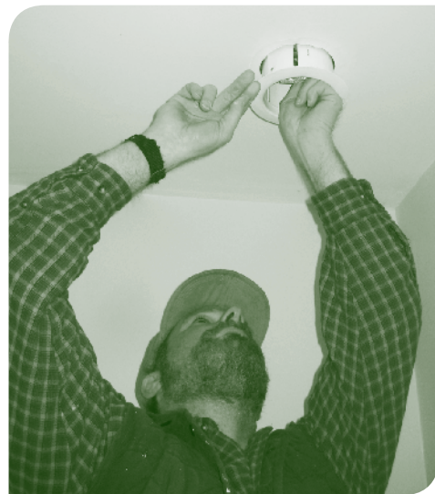
An Arlington HEET volunteer installs an energy-efficient ceiling fixture in Jennifer Norris's home.
