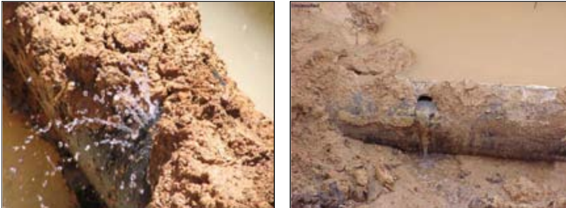
Figure D-16. Fire Protection Lead-In Piping Corrosion.
