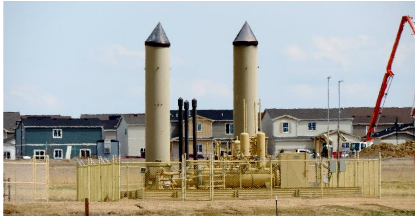
Oil and gas operations in direct proximity to homes in Weld County, Colorado. The current scientific consensus is that a 2,000–2,500-foot setback is needed to protect health and safety, especially that of children. Fossil fuel industry representatives have fought against standards that would keep dangerous oil and gas operations a safe distance from children and families. SOURCE: WildEarth Guardians
