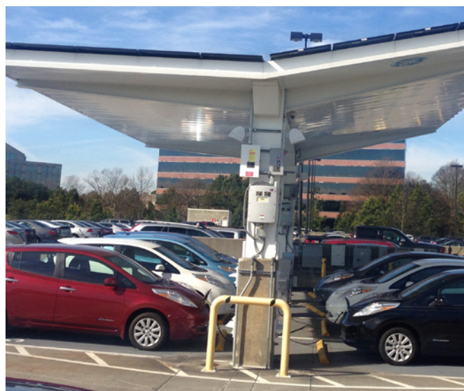
When EVs are charged using renewable electricity—as with this solar charging station in the Atlanta metro area—their overall emissions are equivalent to a gasoline-powered vehicle that gets more than 500 miles per gallon.
