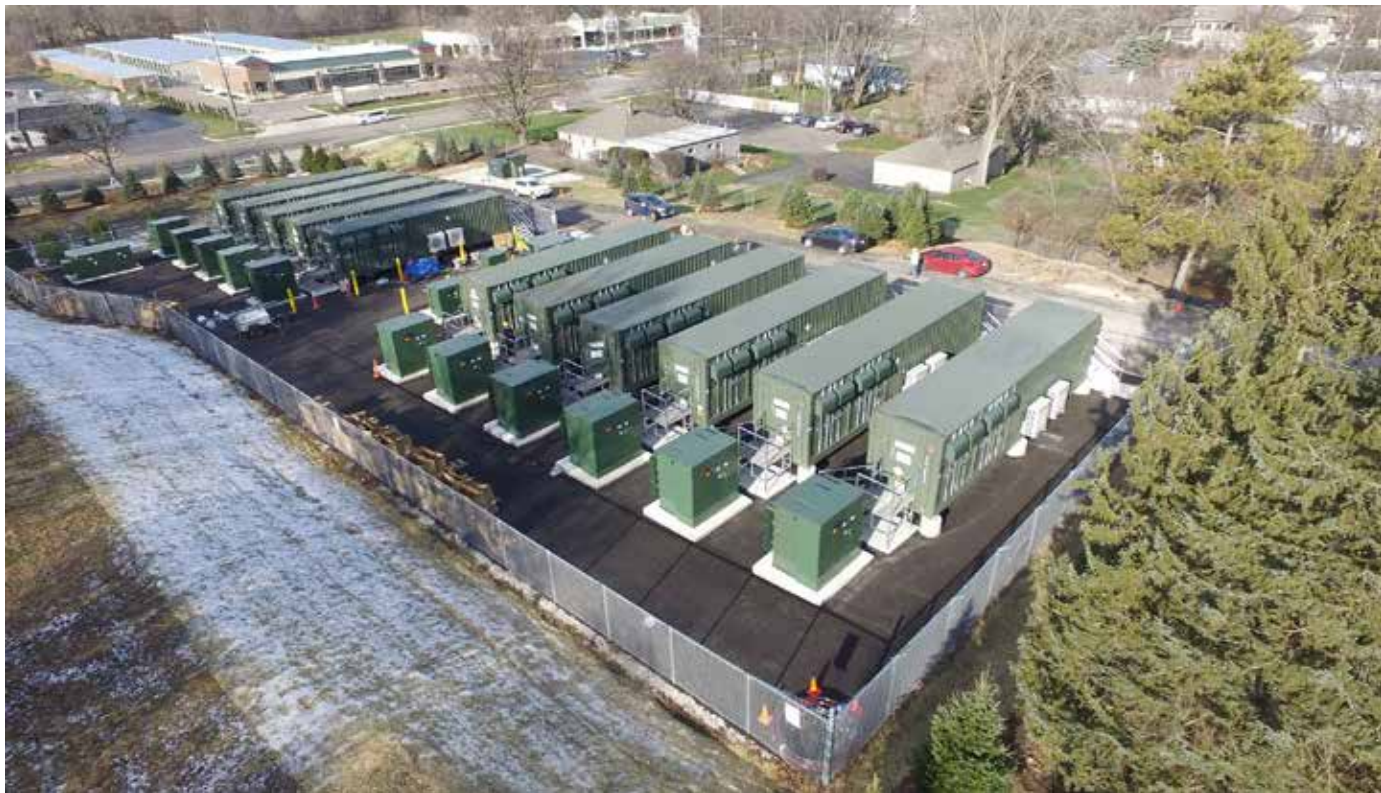
Energy storage, such as this battery storage facility in McHenry County, can be coupled with solar electricity generation to provide a stable supply of electricity to replace existing generation at coal plants.
