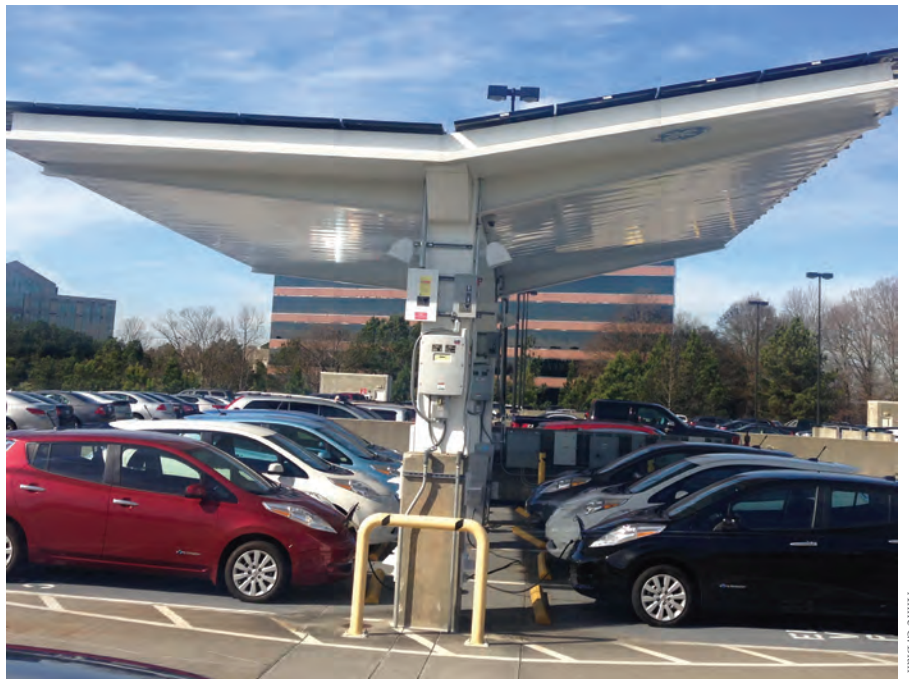
Installing EV charging equipment at office buildings and retail centers can help expand EV ownership by giving more people access to convenient charging options. Workplace charging can also take advantage of high midday solar production.
